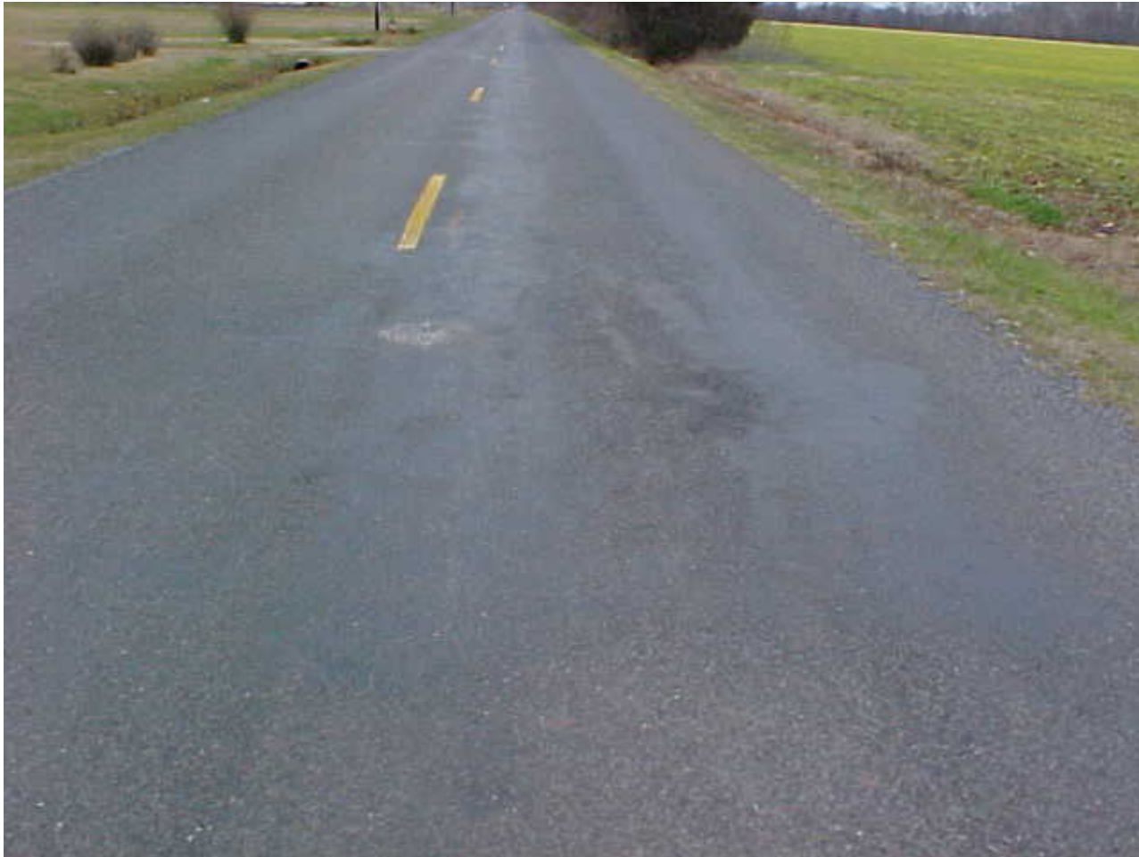
Completed AST Project (Beginning Of Base Failure)
