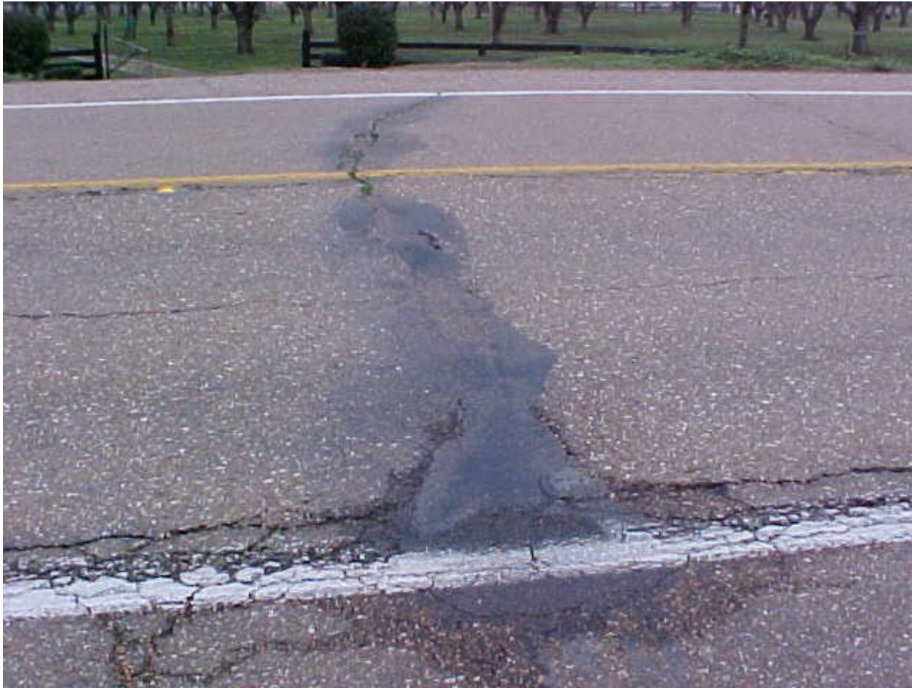
Reflection Of Transverse Joint in underlying PCC Pavement
